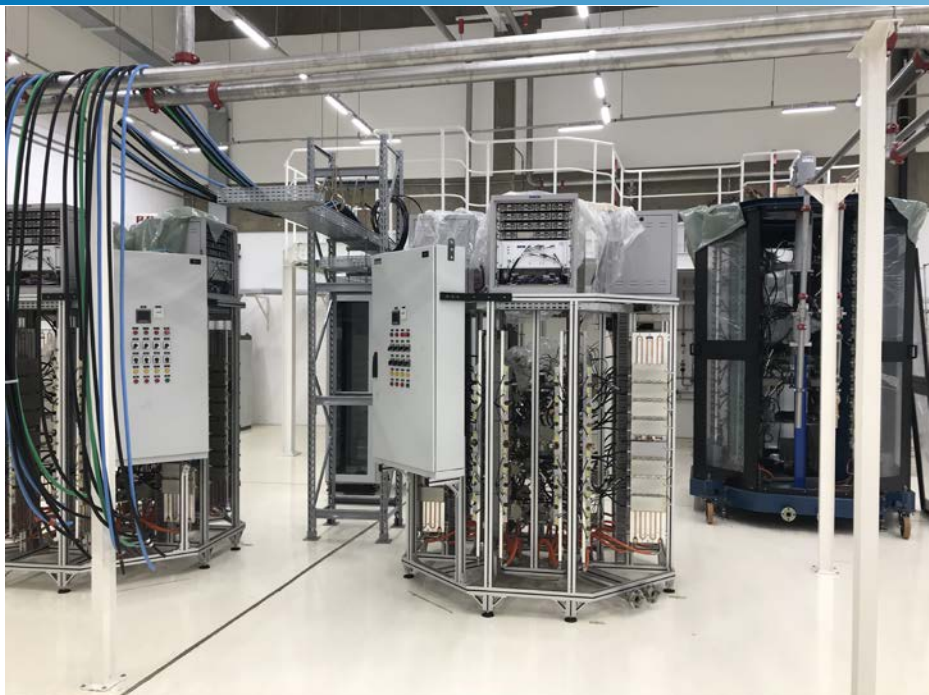
Installation of RF cavity solid state amplifiers
