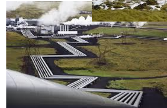
Hellisheidi geothermal power plant Carbfix CO 2 storage project, Iceland
