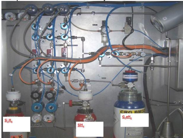
Fig. 3: Photograph of the inside of the gas cabinet.
