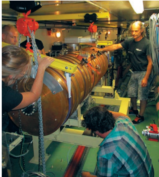
Fig. 159: Members of the RF group manage the tricky installation of two five-cell cavities in the booster.
